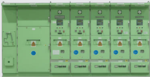
High Voltage Switchboard
