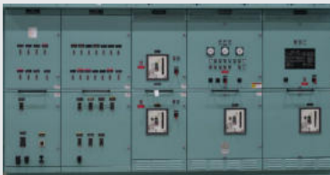
Low Voltage Switchboard
