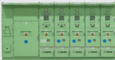
High Voltage Switchboard
